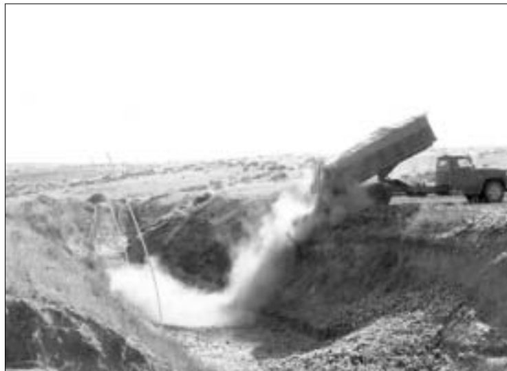
Figure 3. Filling of the pit should begin at one end in order to facilitate coverage with soil during loading.
